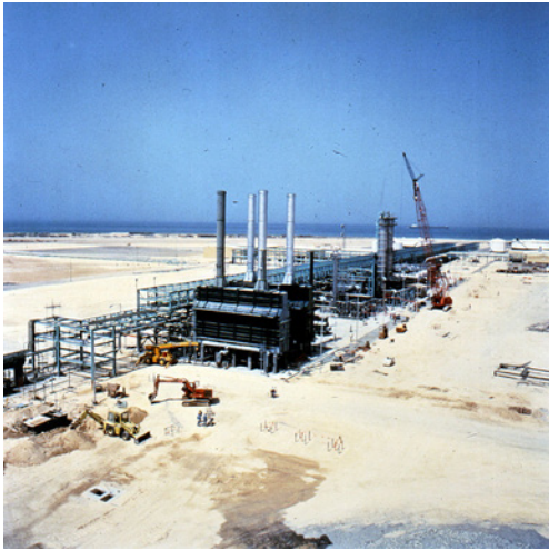
Figure 3-13 Oil refinery construction site of Hyundai Construction Corp. Source: National Archives of Korea.
